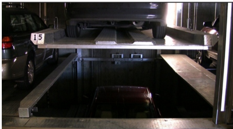
One car below ground and another on a platform that rises up demonstrate how 29 cars can fit in a space normally filled by 10.
